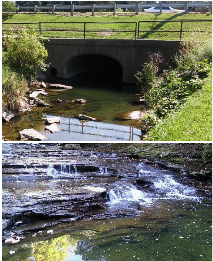
Figure 5. A culvert (top) and waterfall (bottom) along Euclid Creek are fish passage barriers.
